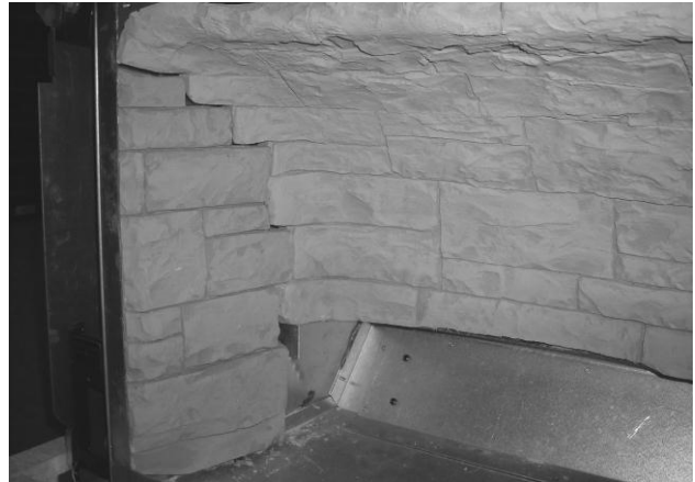
Photo 2 - Left Baffle Panel
